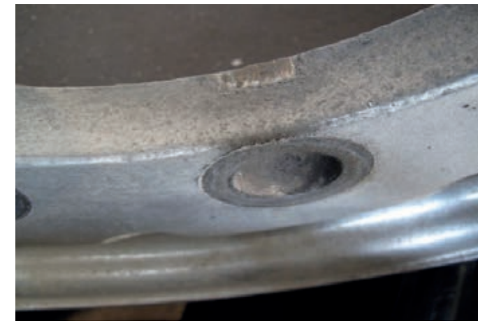
Corrosion wheel nut area and inside bore
