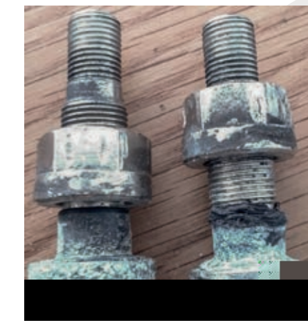
Severely corroded valves
